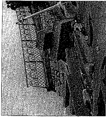
EROSION AT THE SHORELINE
